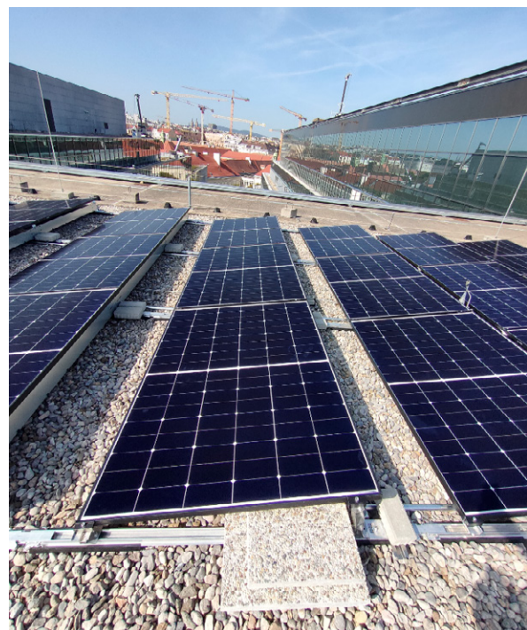
New photovoltaic system on the roof of the OeNB's Money Center in Vienna
